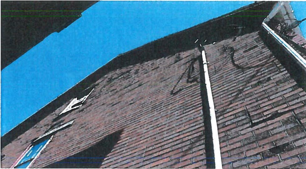
Figure 8. Close-up view of deteriorating imitation brick siding, peeling off of original wood siding in various places.
