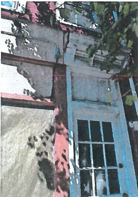
Figure 5. Close-up view of original transom and cornice that will be uncovered and reconstructed, respectively, above the storefront.
