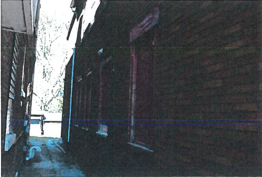
Figure 2. Deteriorating side windows fronting onto alley.
